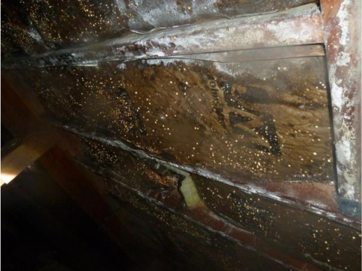
Moisture dripping from the insulation
