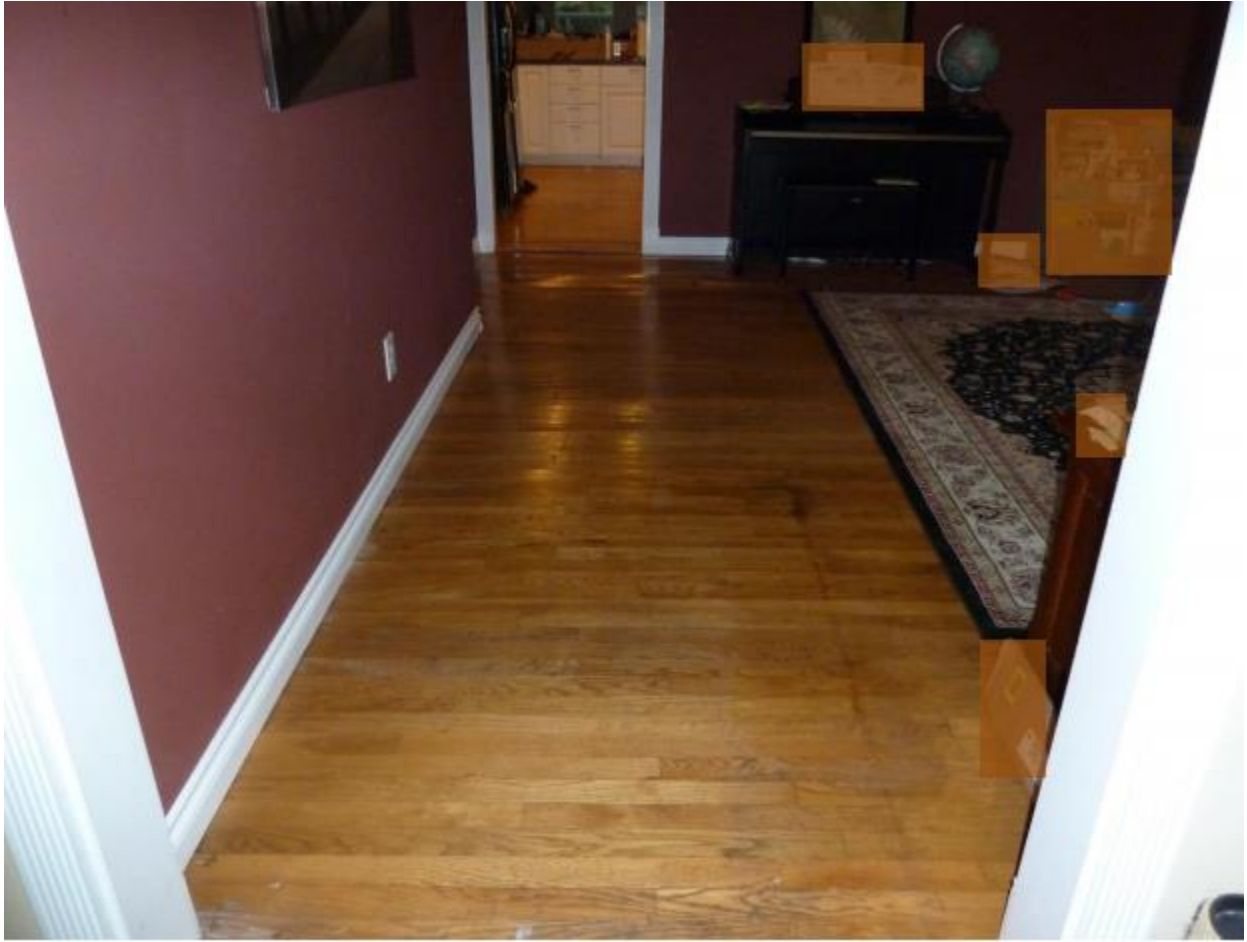
The break is in the kitchen area thru the opening in this picture. The floor was buckled from the opening in the picture all the way to the front door.
