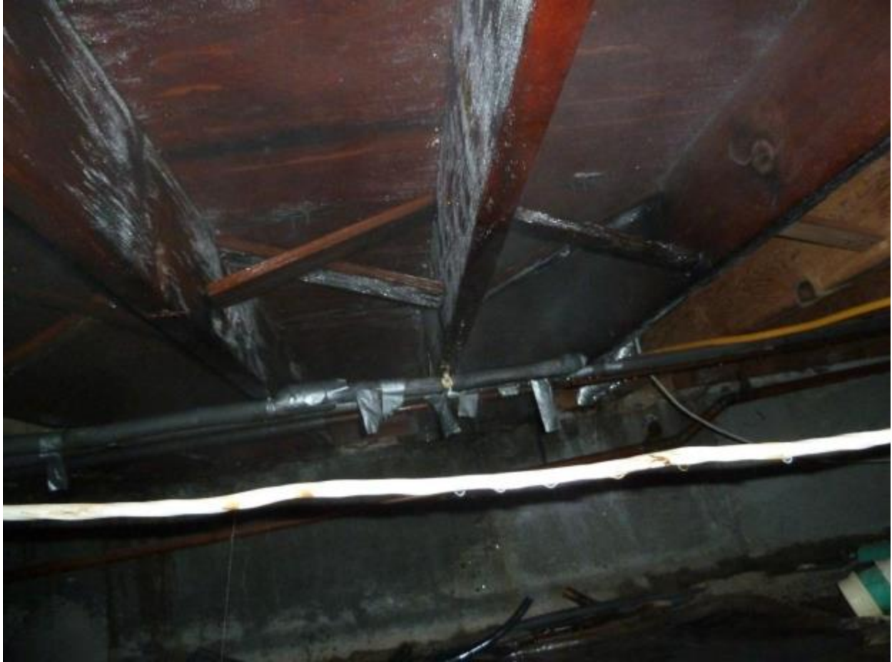
The same area looking over to the pipes. The black wrap is the new pvc line. There is no insulation so the wood really got wet.
